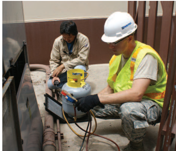
An HVAC professional can inspect and test a furnace to make sure it is operating safely and efficiently. Photograph provided by NAVFAC Hawaii HVAC Specialists
