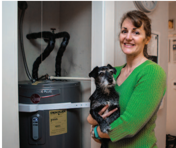
Insulating the first several feet of the hot water pipe where it leaves the tank is an energy saver. Photograph by Marcela Gara, Resource Media, EE Image Database
